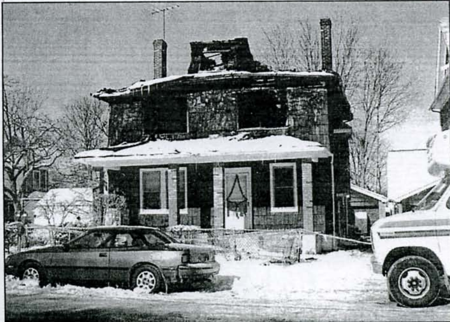
The fire, which broke out just before midnight last Friday night, engulfed the second and third floors of the house, causing a collapse of the third floor as well as the front dormers.
